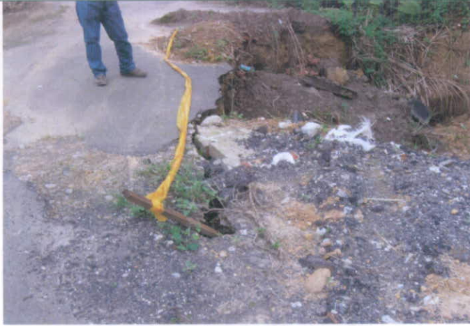
烘內坑煤礦本斜坑塌陷之地表裂縫-1
